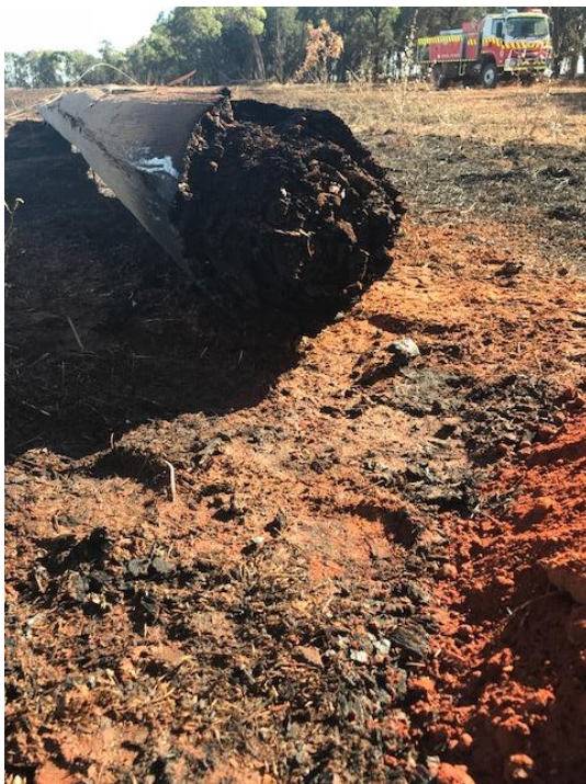
Caption: The base of an Essential Energy power pole following a stubble burn incident on a property in regional NSW.
