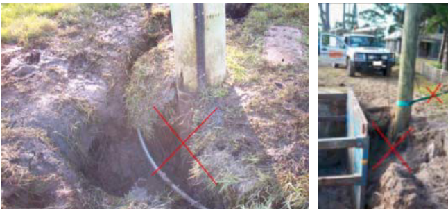
Above: Poles will become unstable if undermined.
